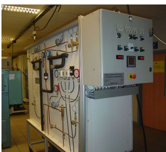
Refrigeration system with control panel and circuit fluid
